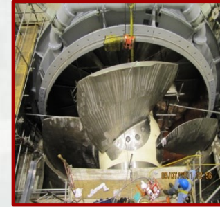
Webbers Falls Turbine
