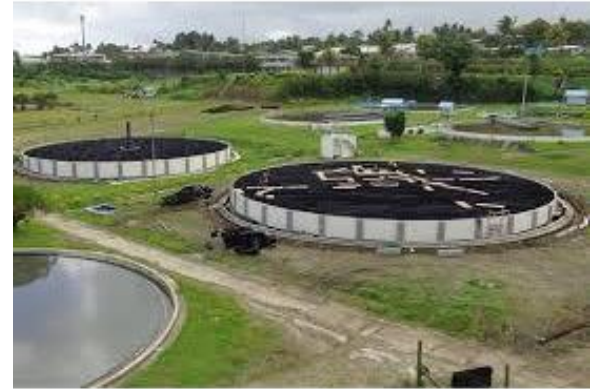
First Treatment Systems – 1950s and 1960s
