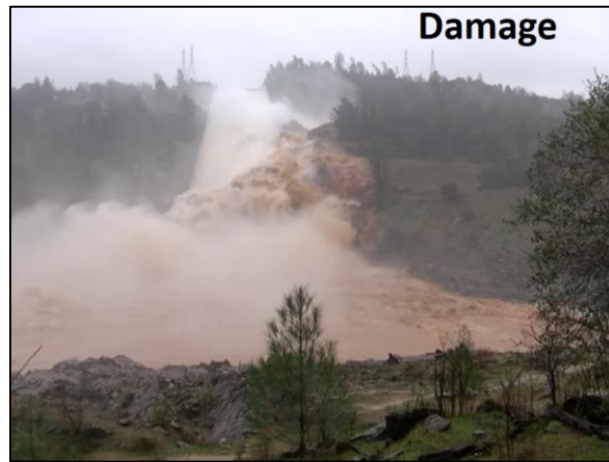
Oroville Dam Spillway Damaged
