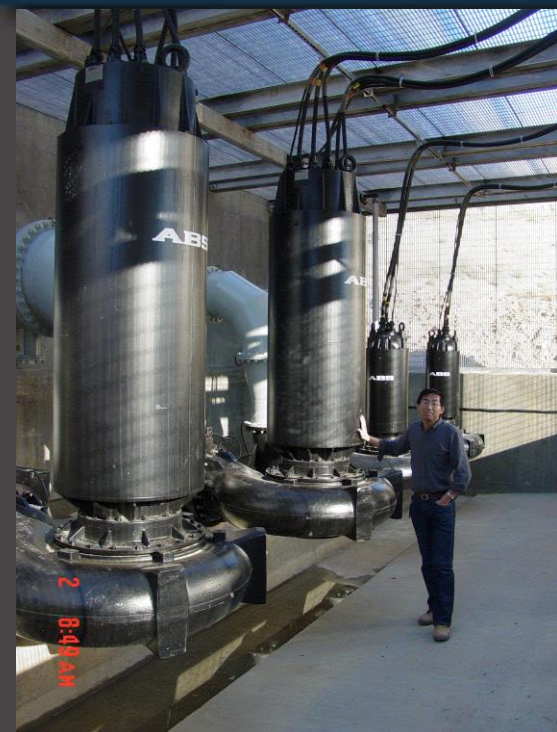
Pump stations and pipelines
