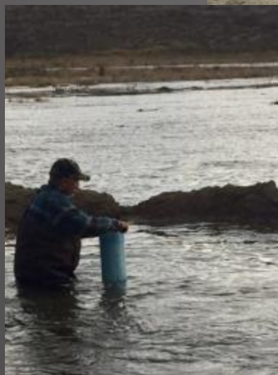
Recharge system operators, instrumentation, and SCADA system
