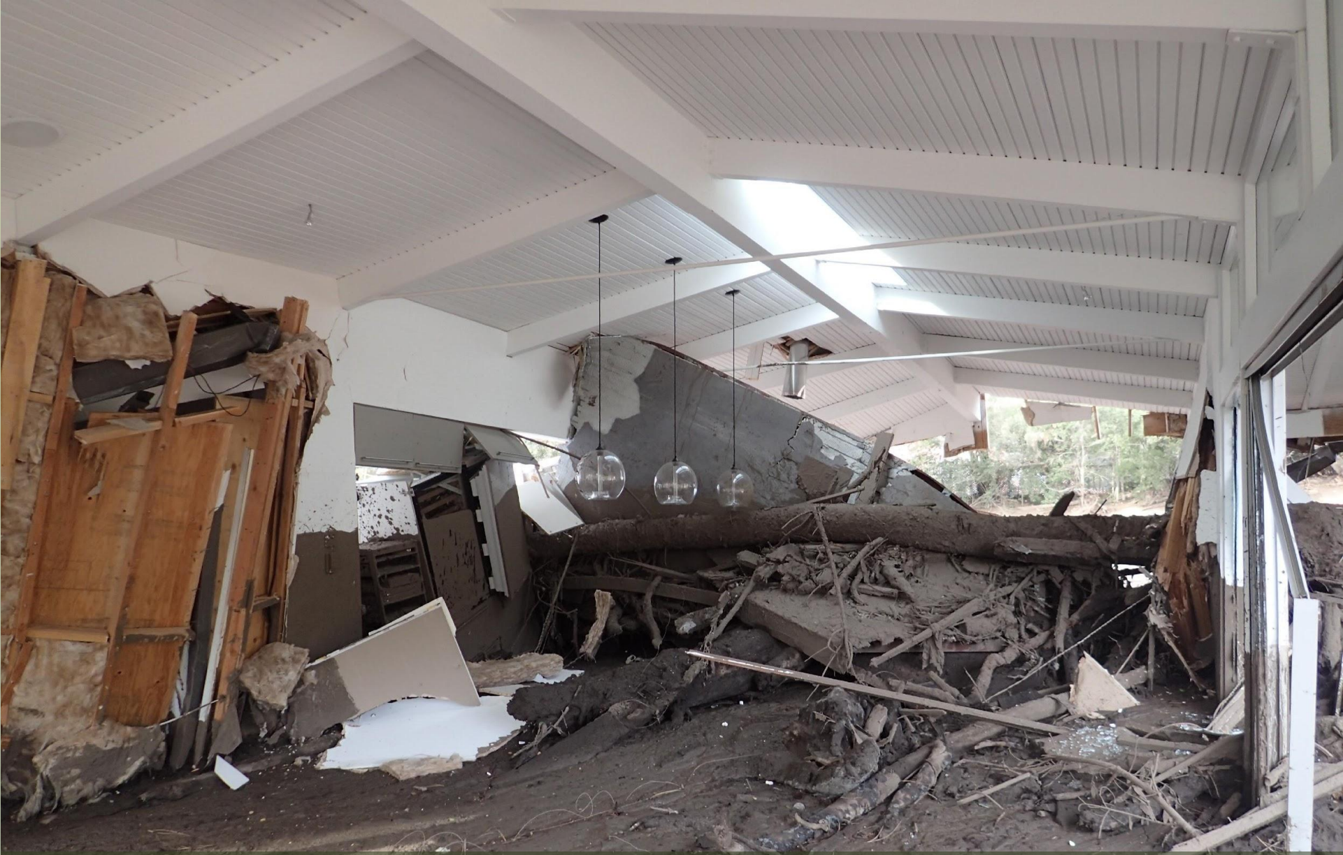
Debris Flow, 2018 Thomas Fire, California
